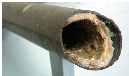
Section of pipe with evidence of limescale
