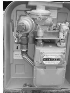
Typical LPG Meter Installation
